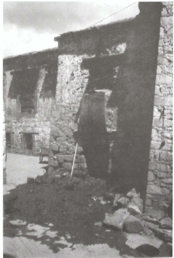
Toilet in conservation area before repair
