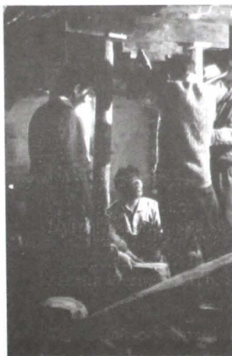
THF workers preparing to change a rotten pillar on the ground floor of Tadongshar House
