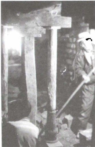
THF workers jacking up a section of Tadongshar to remove the rotten pillar
